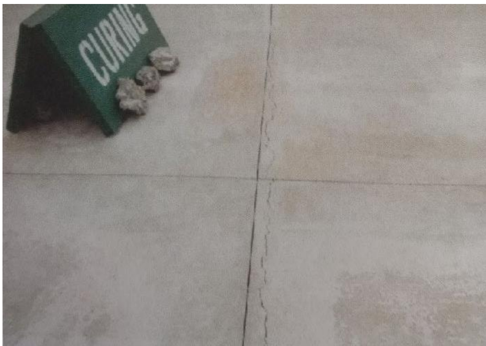
1- picture. Cracks in the seams.
